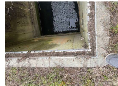
Both grate structures on Foxtrot Taxiway side have 2" inset lip that supports the current aluminum grate.
