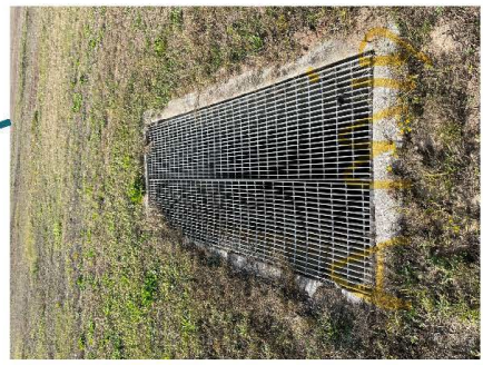
A Mid Field Grate & Location
