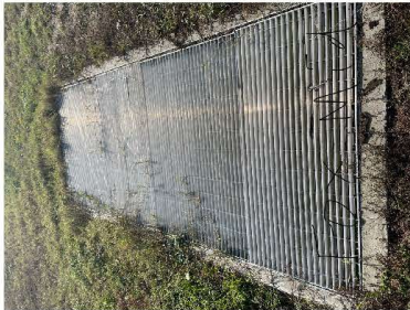
Foxtrot mid field grate & location
